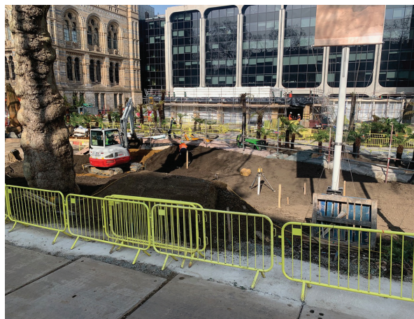
Works in progress outside the NHM: from eastern end to western end, site of the new Urban Garden, March 2024
