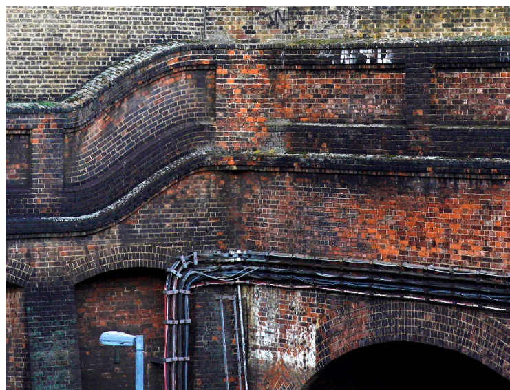
SOPHISTICATED CURVED HISTORIC BRICKWORK (DEMOLITION TO ROAD FRONTAGE IS PROPOSED BY APPELLANT)
